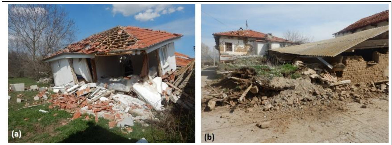
Figure 8(a): Heavily damaged hollow brick structure, (b): Collapsed adobe structure in Kirka village.
