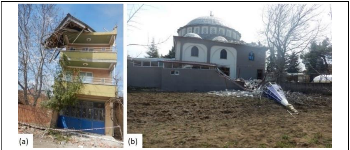
Figure 9(a): Hollow brick built roof floor failure of a reinforced structure. (b): heavily damaged masonry mosque in Oğuz village.
