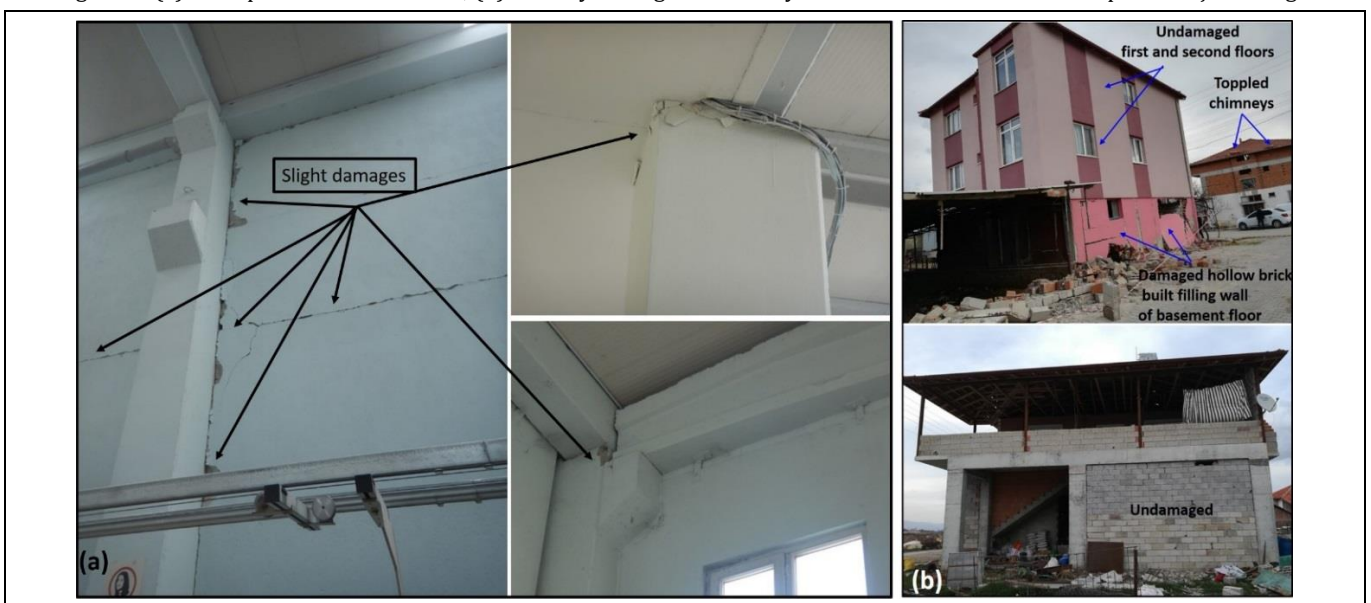
Figure 11(a): Damages on precast concrete modern textile factory structure in Yassihüyük village, (b): Partly damaged three-storey reinforced structure and undamaged single-storey reinforced structure in Apa village.
