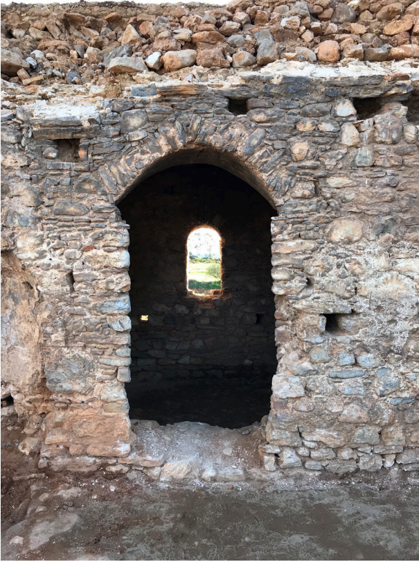
Fig. 10: Doorway leading into U04, showing springing of the supporting arch and holes for tie beams (2018).
