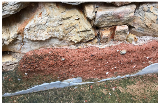
Fig. 20: After cleaning work (December 2018) – a: Northwest corner of U07, layers of plaster; b: Thick plasters with high content of brick powder from the west wing; c: used as bedding for marble facing at the Early Byzantine monastery complex in Torba (2018).
