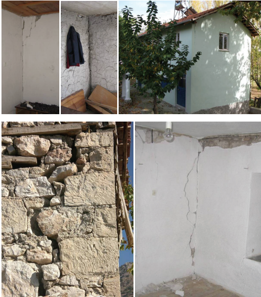
Fig. 11. Damages observed at connection of crossing walls.
