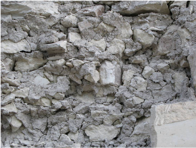
Fig. 8. Bad profile of a damaged wall.
