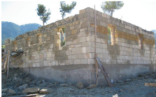
Fig. 12. Damaged building during its construction without partition walls.
