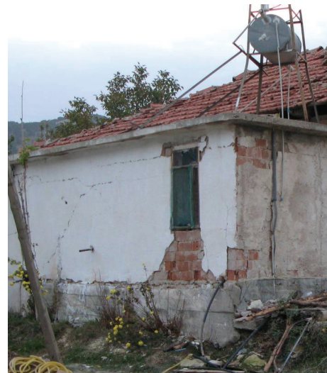
Fig. 14. Damage concentrated around wall opening near the building corner.
