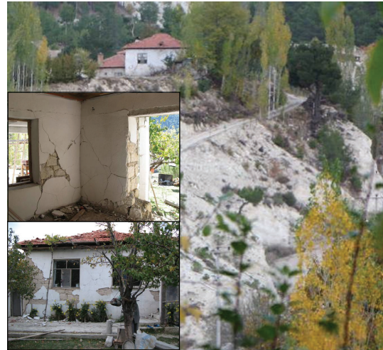
Fig. 17. Damaged building due to slope/hill affect.
