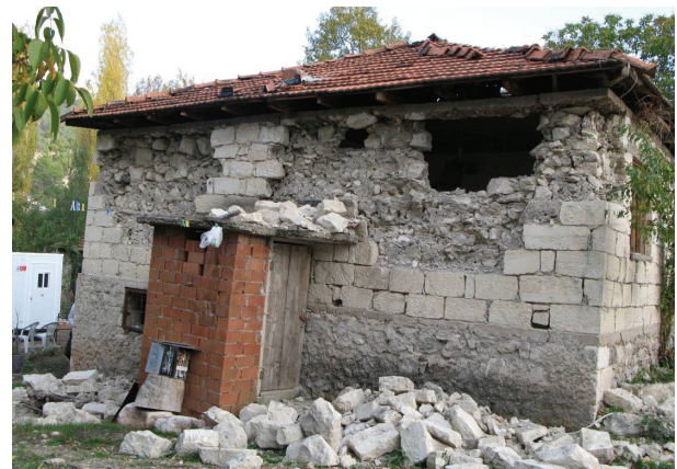
Fig. 7. Typical damage pattern in Çameli earthquake.
