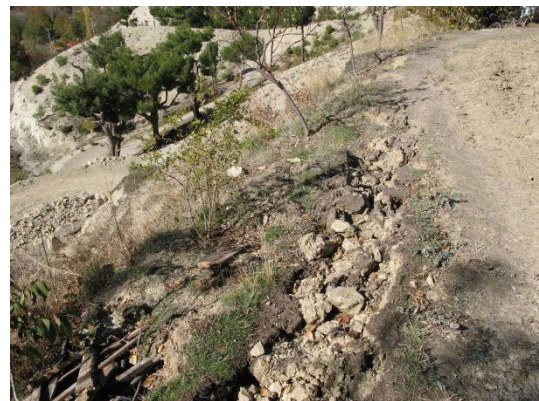
Fig. 18. Cracks on the ground at top of hillside.
