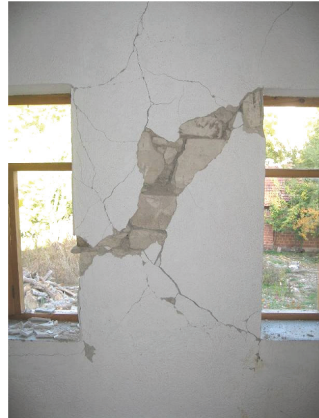
Fig. 13. Damage between two wall openings.
