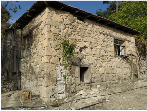
Fig. 15. Out of plane failure due to lack of bond beam.
