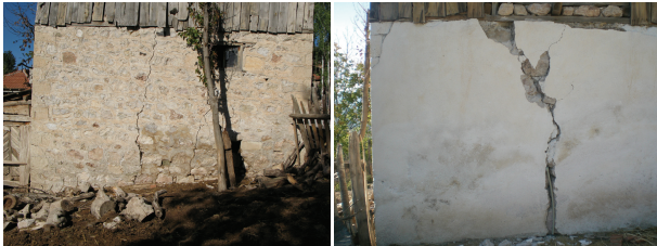
Fig. 16. Out of plane failure due to long unsupported wall length.
