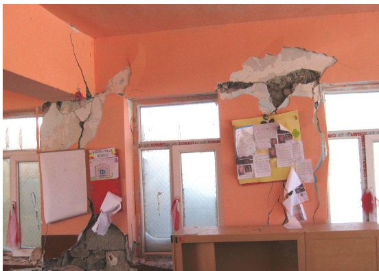
Fig. 10. Damage between two wall openings.
