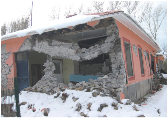
Fig. 12. Out of plane failure.
