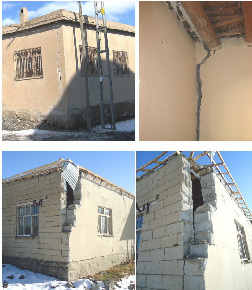
Fig. 9. Damages observed at intersection of outer walls.
