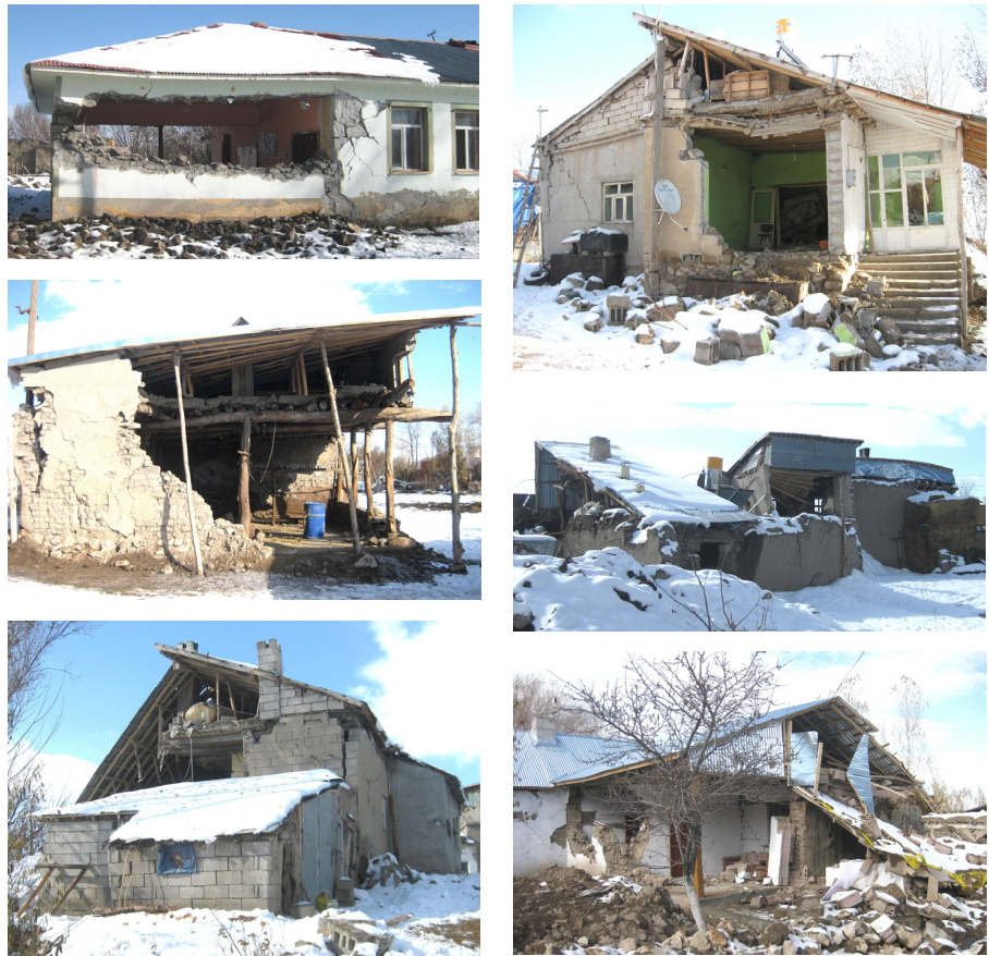
Fig. 5. Various types of damages observed at URM buildings after the 2011 Van earthquakes.
