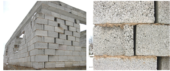
Fig. 14. Wall damage due to low strength joint adhesive.
