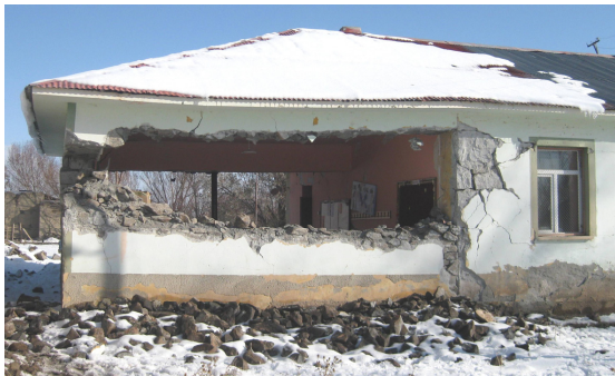
Fig. 13. Out-of-plane failure due to long unsupported wall length.
