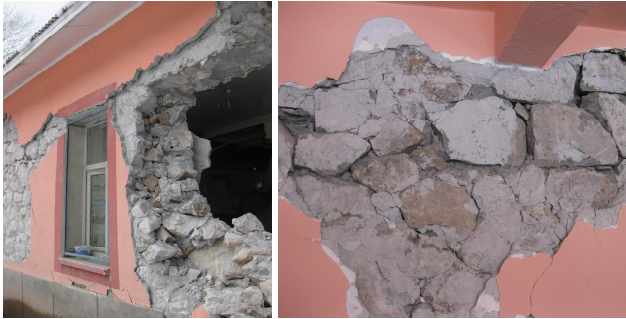
Fig. 6. Profile of a poorly constructed damaged wall.
