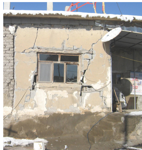
Fig. 11. Damage concentrated around wall opening near the building corner.
